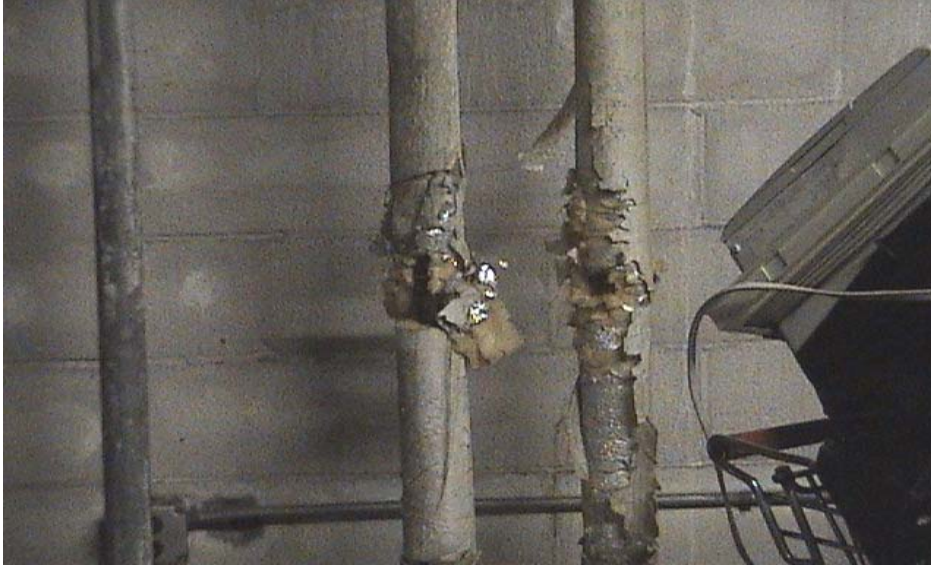
Figure IV. Leaky Pipes and Water Damage to Walls
